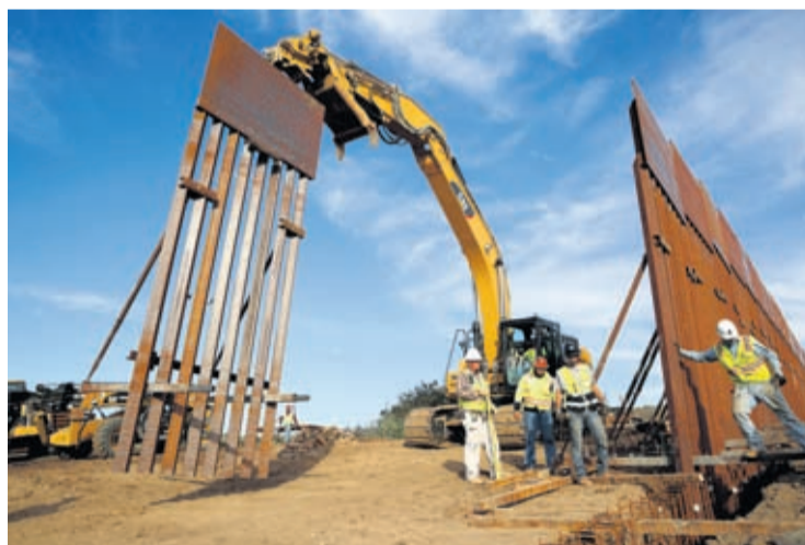
In this Jan. 9, 2019 file photo, construction crews install new border wall sections seen from Tijuana, Mexico.
